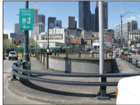
The triangle opening between 2nd Ave Ext S and 4th Ave S
