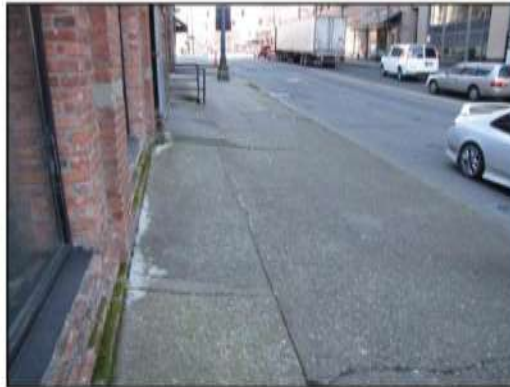
Uneven sidewalks on S Jackson
